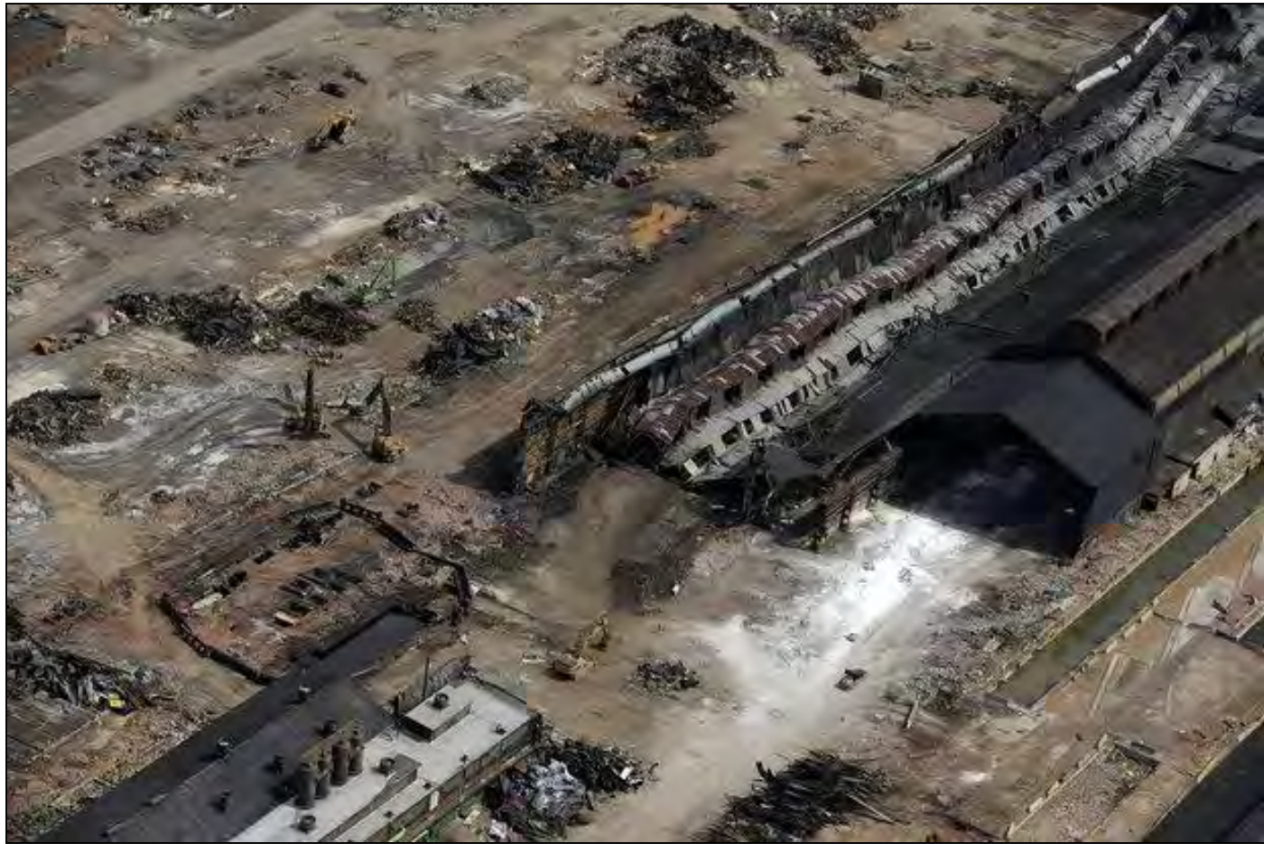
Building collapses during demolition May 5, 2014 Photo by Algerina Perna— The Baltimore Sun
